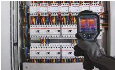
Electric Panel Inspection
